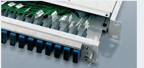
FO Patch Panel
